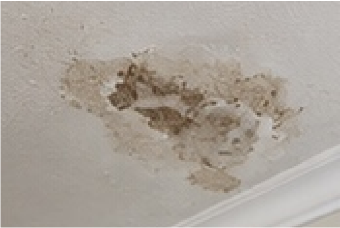
Existing damage · 8:42 am
